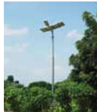
Solar Streetlighting systems (SSLS)
