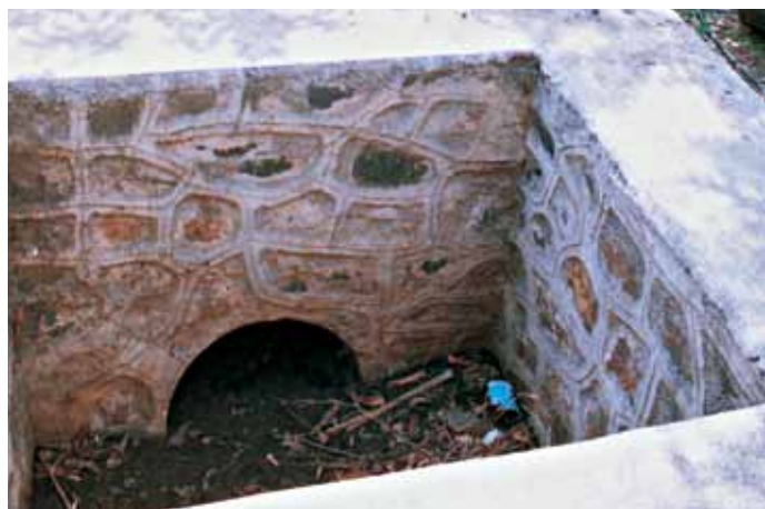
'Rib-loc' pipes: Sub-soil drainage chamber at Jain Hills-Bottom.
