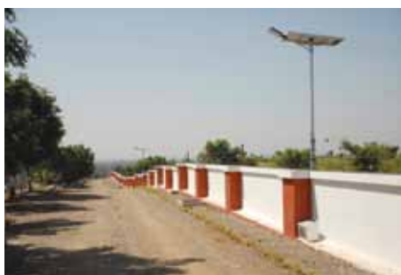
Different Installations of solar power fencing
