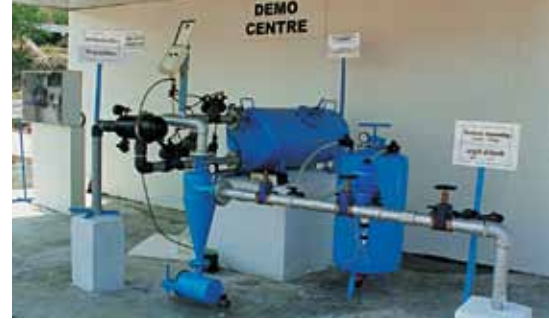
Fertigation station along with venturi assembly
