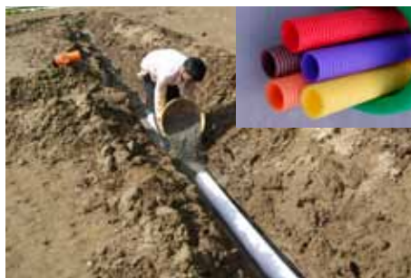
Drainage work in progress near guest house; inset: corrugated pipe used for drainage
